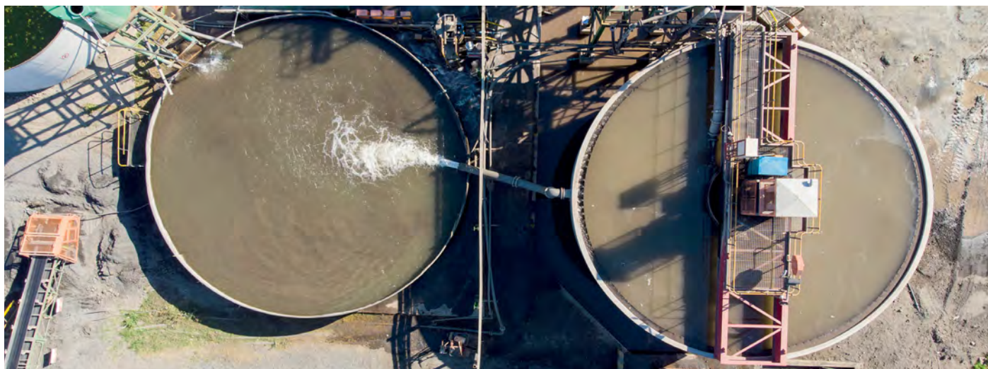
South Africa Windsor 8 water treatment.
