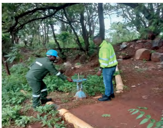
Zambia_Roan water supply to the community
