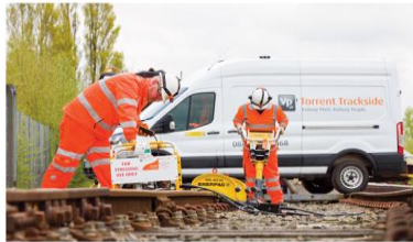
Vp Torrent Trackside Railway Plant. Railway People.
