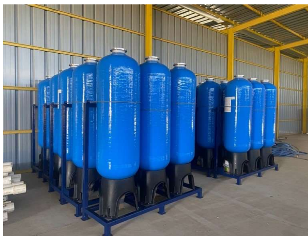
Fig. 8 DLE pilot plant columns installed in Copiapó
