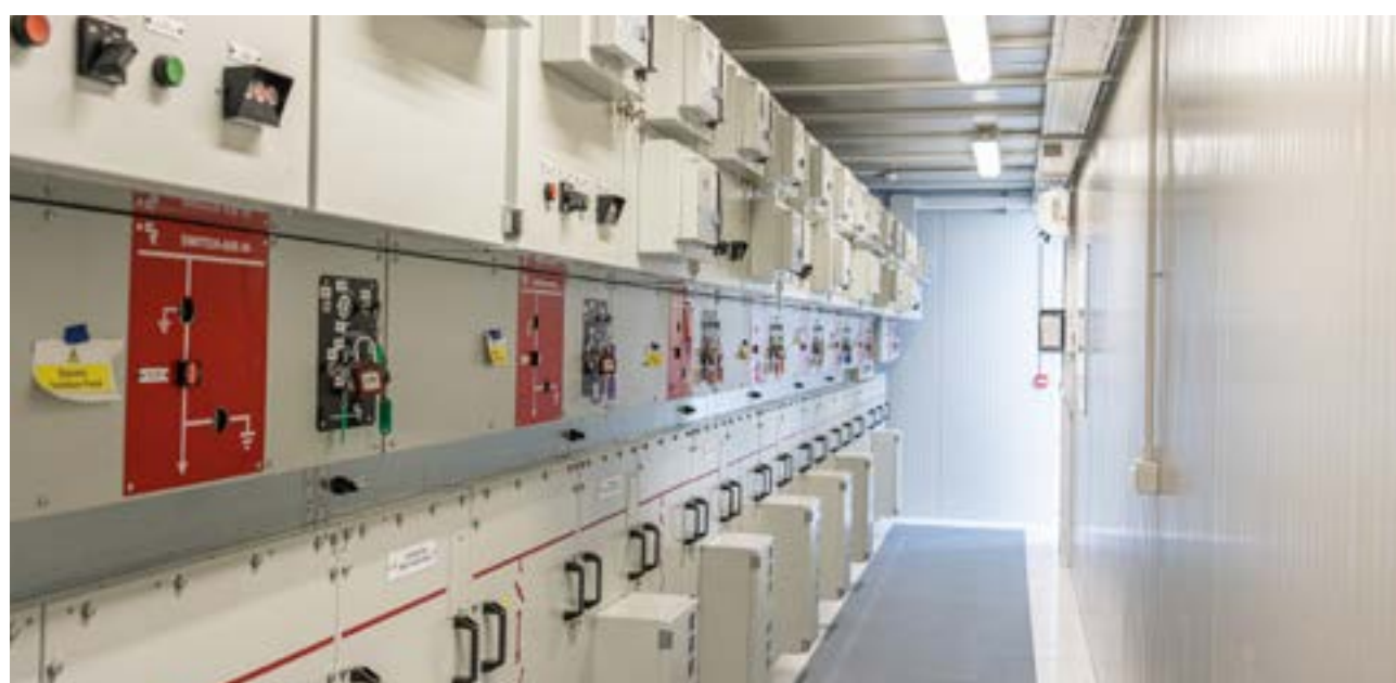
A shot of the control room of the Pillswood project, tracking one of GB's best performing BESS of 2023.
