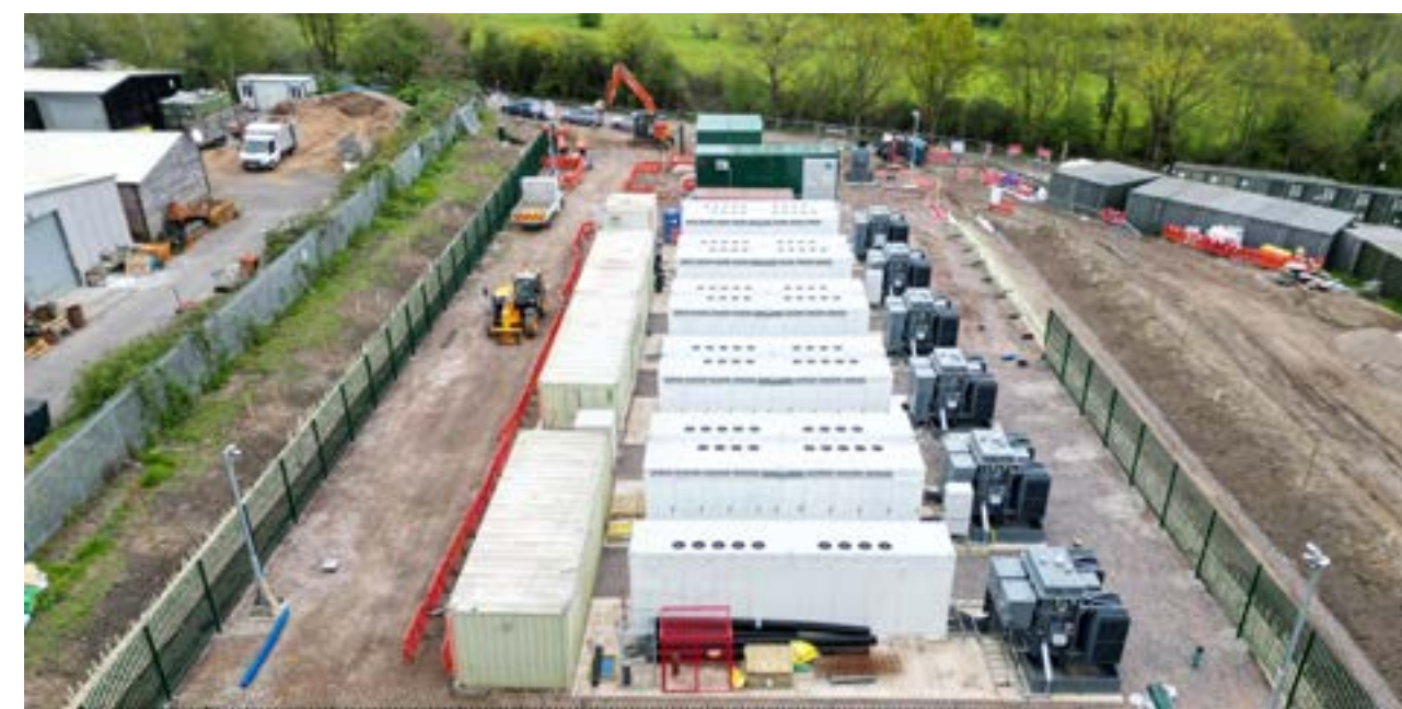
Energised in May 2023, the 20 MW / 40 MWh Farnham Project is the third to be energised in the Company's portfolio.
