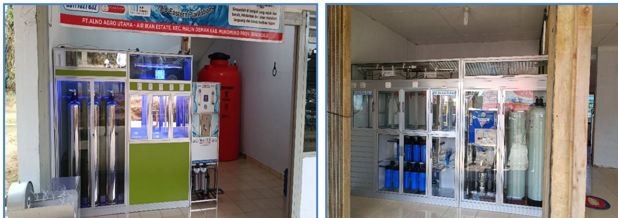
Providing clean water to employees through reverse osmosis
