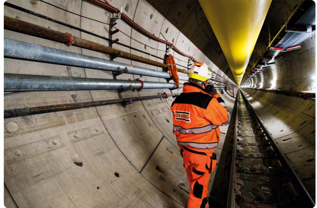
Construction progress of the material transport tunnel that will connect the Woodsmith mine site to the materials handling and port infrastructure.
