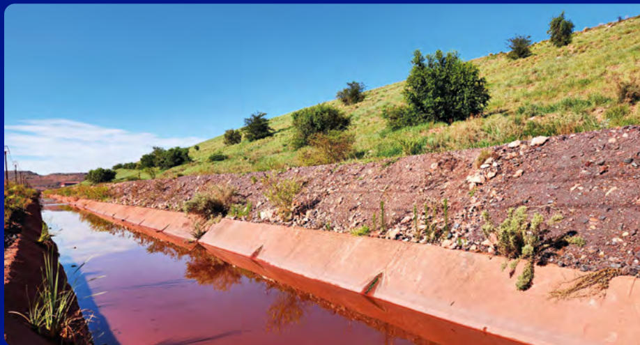
One of the stormwater channels that has been constructed at Sishen to divert excess water away from the mine site.
