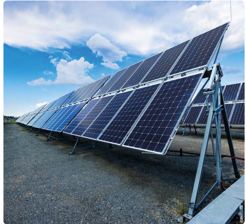
This new solar plant, and the hydrogen plant (nearing completion) it will supply, is making Mogalakwena a strategically important centre for hydrogen production in South Africa's developing hydrogen valley.
