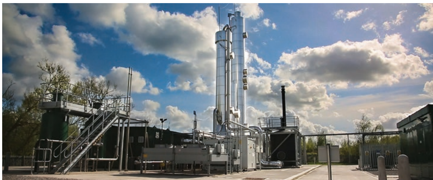
Biomethane Upgrading Plant at Minworth
