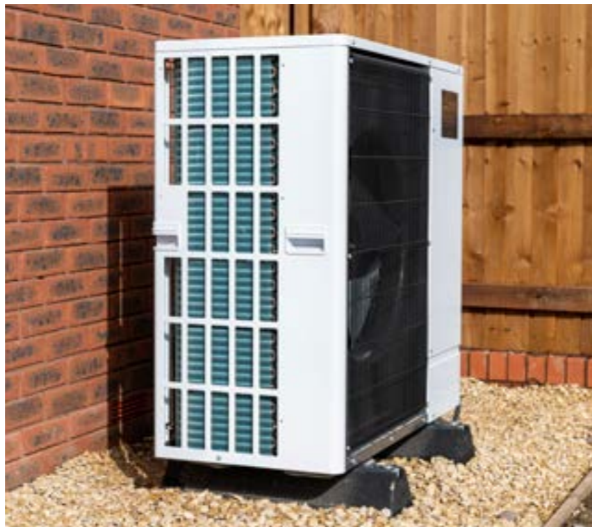
Air Source Heat Pump at Great Milton Park, Newport, Gwent
