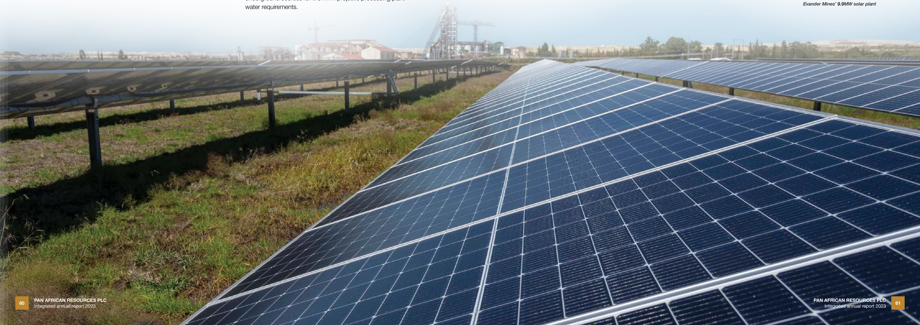
Evander Mines' 9.9MW solar plant
