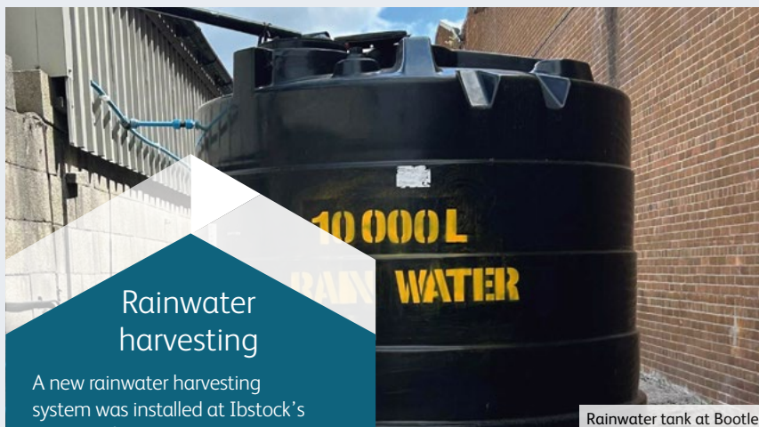
Rainwater tank at Bootle
