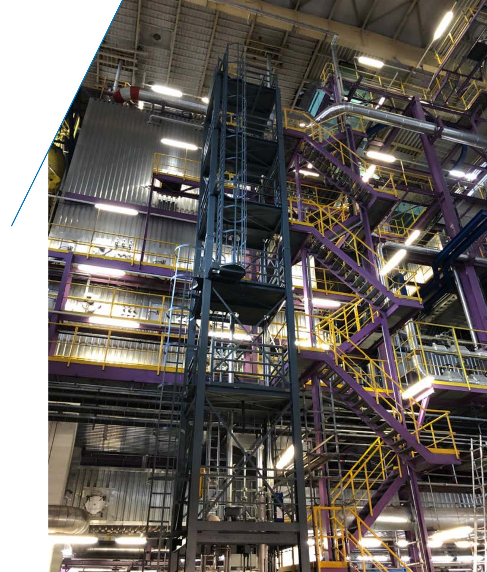
ANDRITZ has supplied its first carbon capture plant to the steel industry. The pilot plant started operating at voestalpine's steel mill in Linz, Austria, in the second quarter of 2023. The plant separates carbon dioxide from the flue gases resulting from iron making using an amine-based process.
