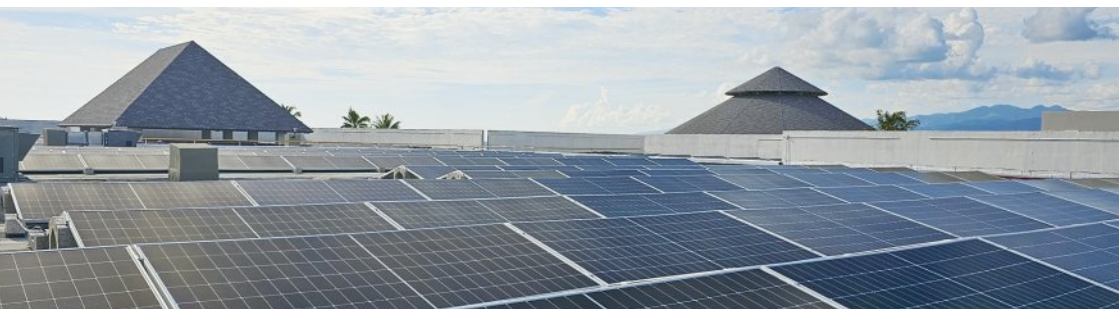
Photovoltaic system at Meliã Trinidad Hotel, Sancti Spíritus, Cuba
