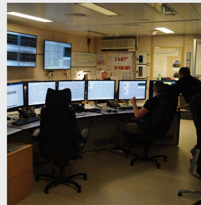
The control room aboard EnQuest's Kraken FPSO
